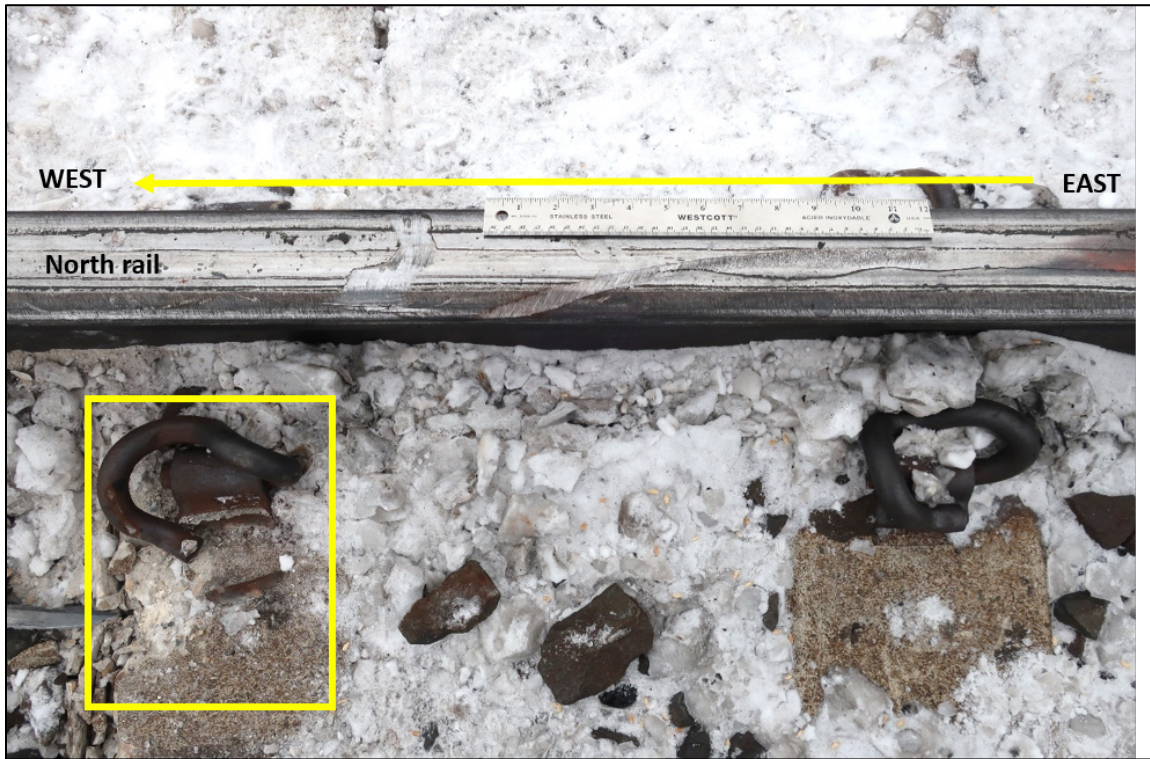
Figure 5. Wheel marks on the top of the north rail and the damaged gauge-side track fastener and tie (shown in the box) at Mile 166.33 (Source: TSB)
