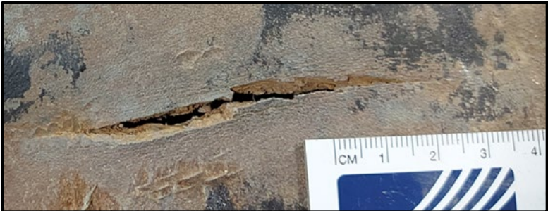
Figure 6. Breach point on NPS 16 line pipe (Source: Acuren)
