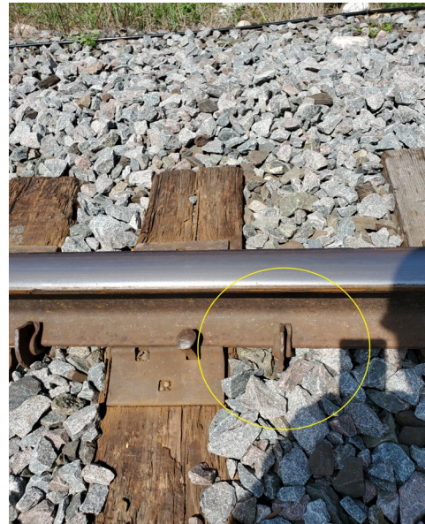
Figure 4. Track in the siding adjacent to the point of derailment, showing an anchor displaced several inches away from the tie (Source: TSB)
