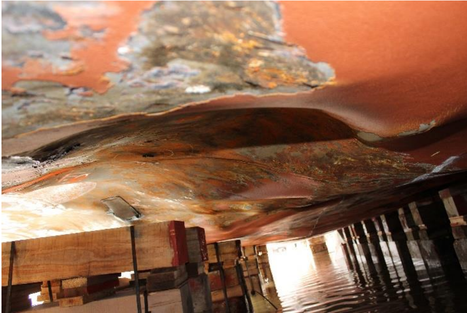
Figure 8. View of hull bottom shell plating deflections, breaches, and temporary repairs carried out by the divers off the Astronomical Society Islands (Source: TSB)
